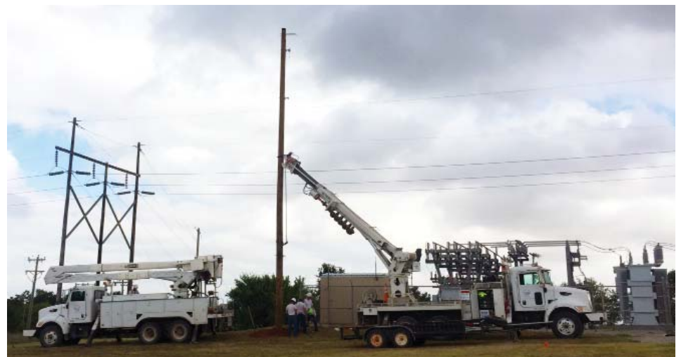
Work continues on installing REC's new metering system. The new system requires seven collector sites. The poles needed for the equipment are being set.
