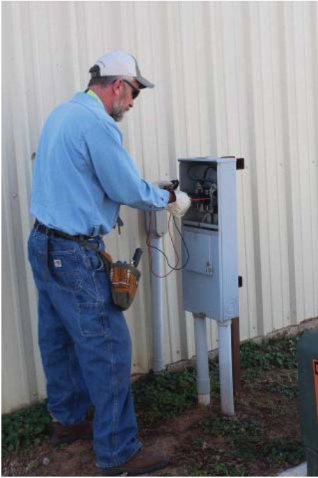
Terry Hall, installer for Chapman Metering, conducts hot socket test before installing REC's new RF meter.
