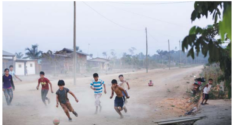
Children in Dos de Junio, Bolivia play soccer at dusk after volunteer linemen from Missouri and Oklahoma finish their work for the day installing power lines in their village.
